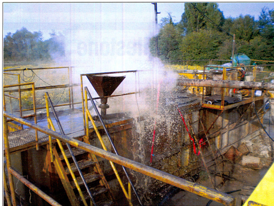
Hot geothermal water from the first geothermal evaluation well in Szentlőrinc, Hungary. (Image courtesy of KMS Technologies – KJT Enterprises Inc.)
